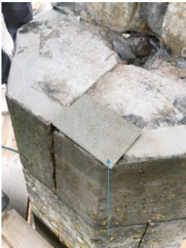
Base of the corroded iron rod ended in a pocket 5 courses below the cross. Sample of Crosland Hill sandstone, (grey/ buff ) adjacent to face stonework.
