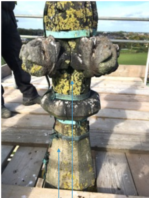
Vertical cracks through the top two pinnacle stones
